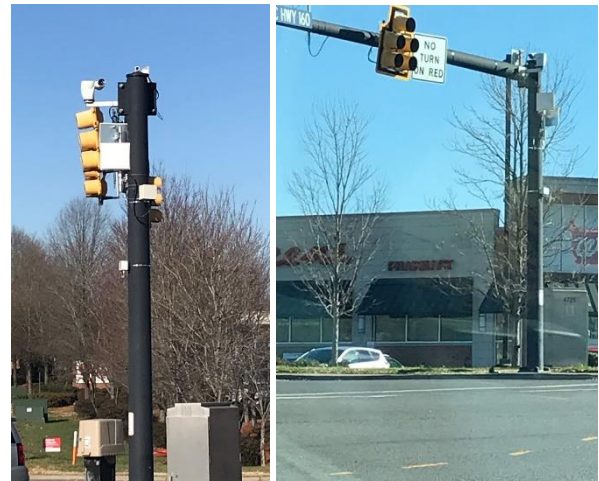
Adaptive Traffic Signal at SC 160 and Sutton Road/Pleasant Road
